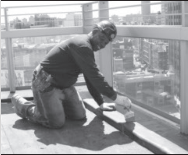
Contact adhesive is applied to the flashing by Local 8 Journeyman Charles McDougle.
