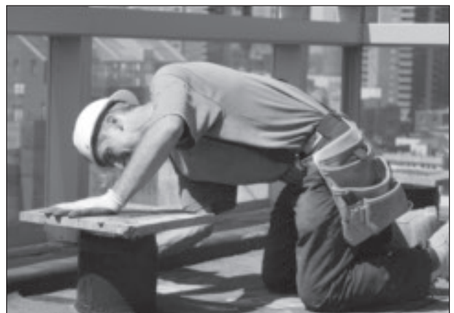
Local 8, New York, NY, Journeyman Matthew Mannino prepares to install flashing at One York Street.
